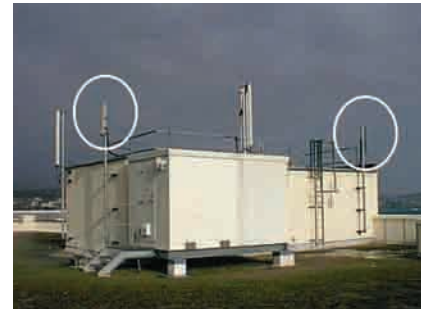
Second and third Generation equipment on a rooftop site. The 3G equipment is highlighted.
