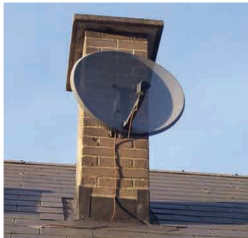
Chimney Mounted Satellite dish.
