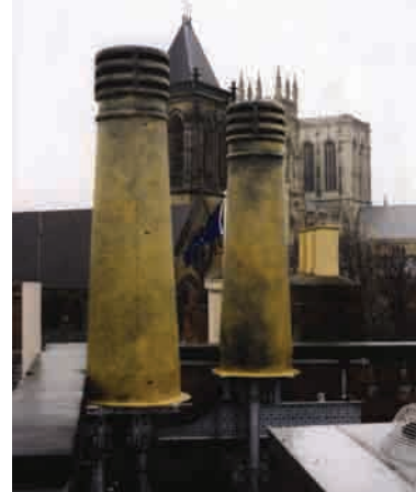
Equipment disguised as a chimney pot.
