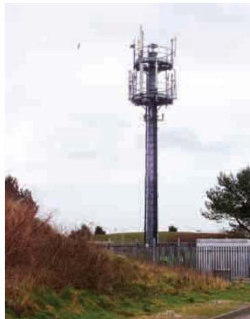
A mast located at a wastewater treatment site
