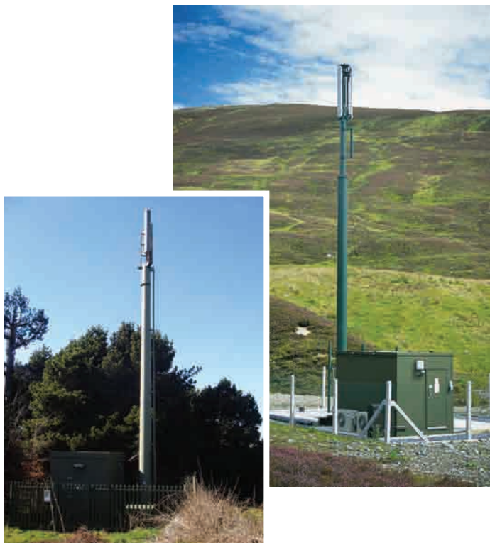
Examples of masts and ancillary apparatus painted to minimise contrast with the surrounding environment.
