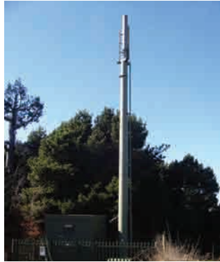
Equipment cabinet adjacent to a monopole mast.
